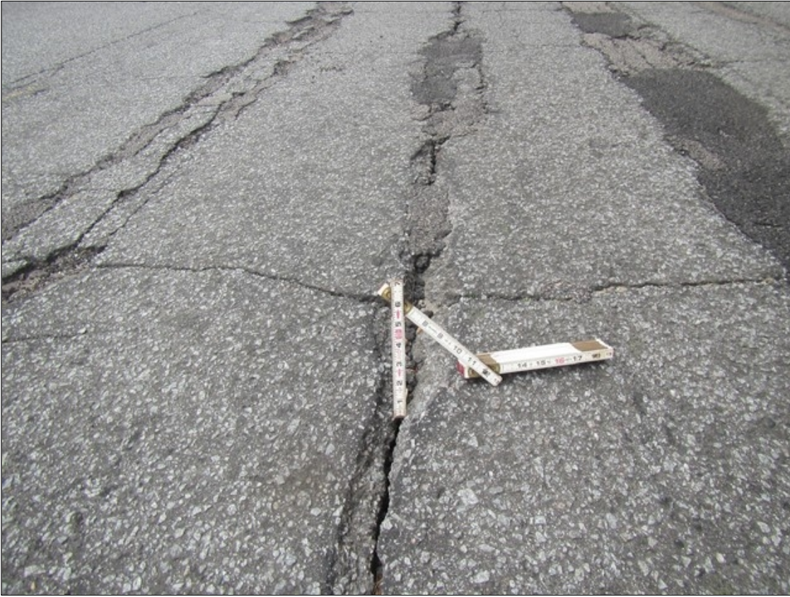
Span 1 Wearing Surface: MUNICIPAL PAR: 22 FOOT X 8 FOOT AREA WITH UP TO 3/4 INCH SETTLEMENT, FAILED PATCHES UP TO 17 FOOT LONG X 15 INCH WIDE WITH 1/2 INCH ALLIGATOR CRACKS AND POTHoles UP TO 14 INCH X 8 INCH X 2 INCH DEEP THROUGHOUT WESTBOUND LANE
