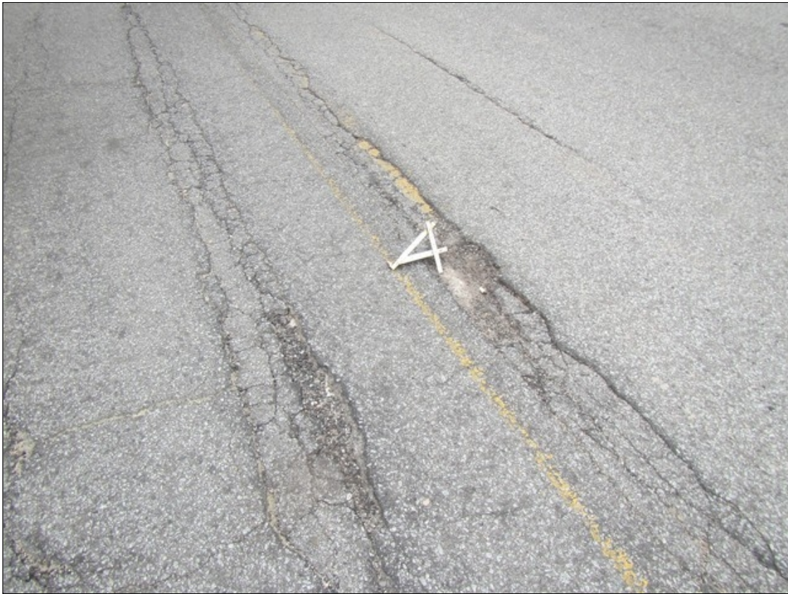
Span 1 Wearing Surface: MUNICIPAL PAR: IN EASTBOUND LANE NEAR MIDSPAN, 15 FEET X 3 FEET AREA OF UP TO FULL DEPTH POTHOLING ALONG BEAM EDGES
