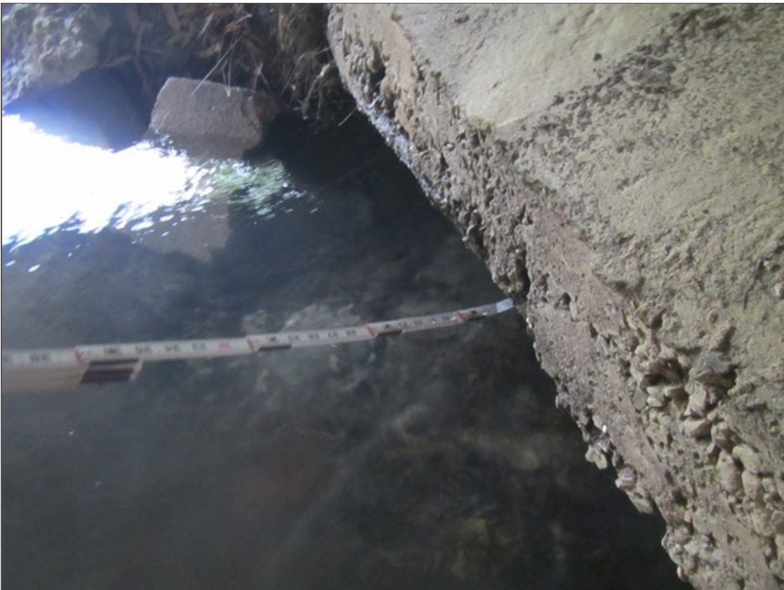
End Bent 1 Abutment: MUNICIPAL PAR: 10 FEET X 1 FEET DEEP SCOUR WITH 2 FEET DEEP UNDERMINING UNDER ABUTMENT UNDER UNIT 13-15
