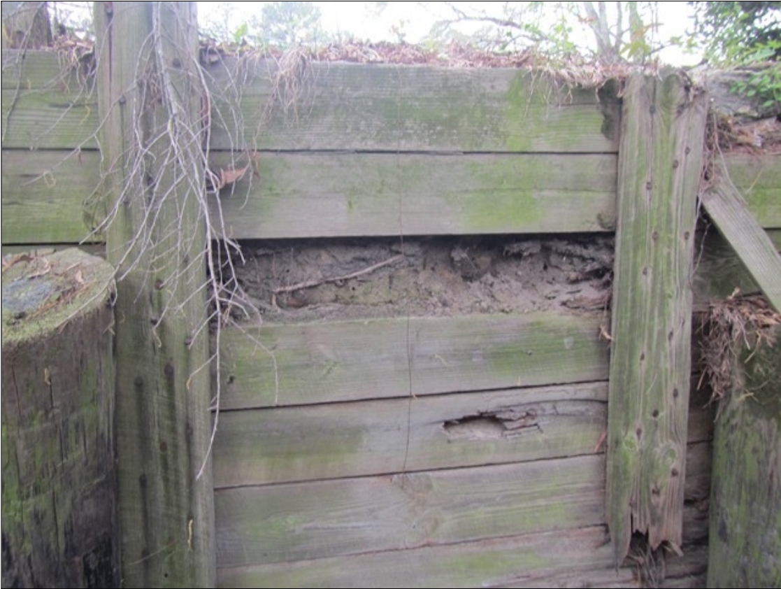
MUNICIPAL PAR: 55 INCH X 9 INCH X FULL DEPTH AREA OF DECAY WITH EXPOSED FILL IN FACE OF NORTHWEST WINGWALL APPROXIMATELY 2 FEET FROM TOP OF WINGWALL
