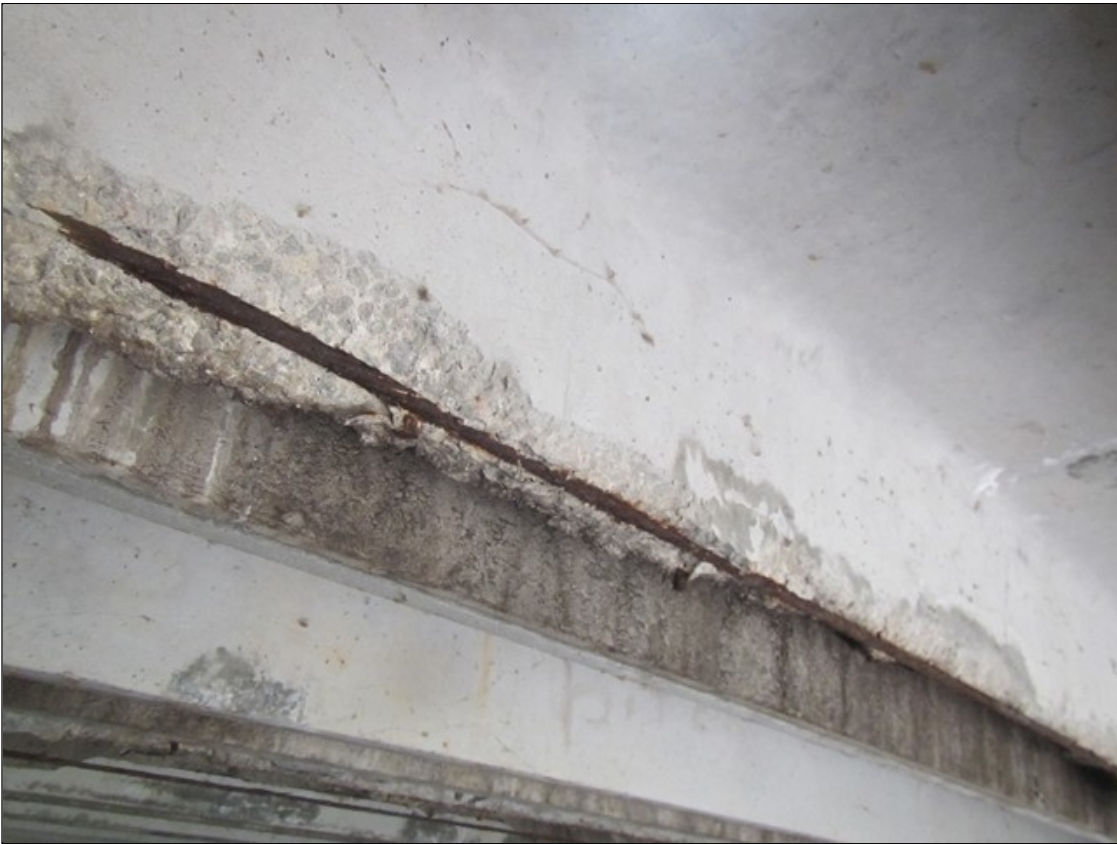
Span 1 Slab 4: MUNICIPAL PAR: (2) SPALLS WITH EXPOSED REBAR AND STRANDS UP TO 7 FOOT X 3 INCH X 4 INCH IN LEG 2, APPROXIMATELY 7 FOOT AND 10 FOOT FROM ABUTMENT 1
