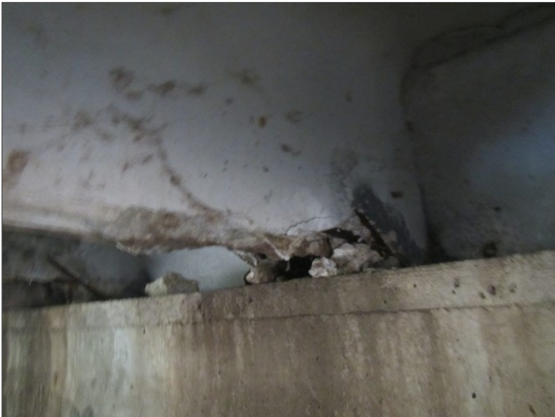
Span 1 Slab 15: MUNICIPAL PAR: 20 INCH X 3 INCH X 3 INCH SPALL WITH EXPOSED REBAR AND STRAND IN LEG 2 AT ABUTMENT 1
