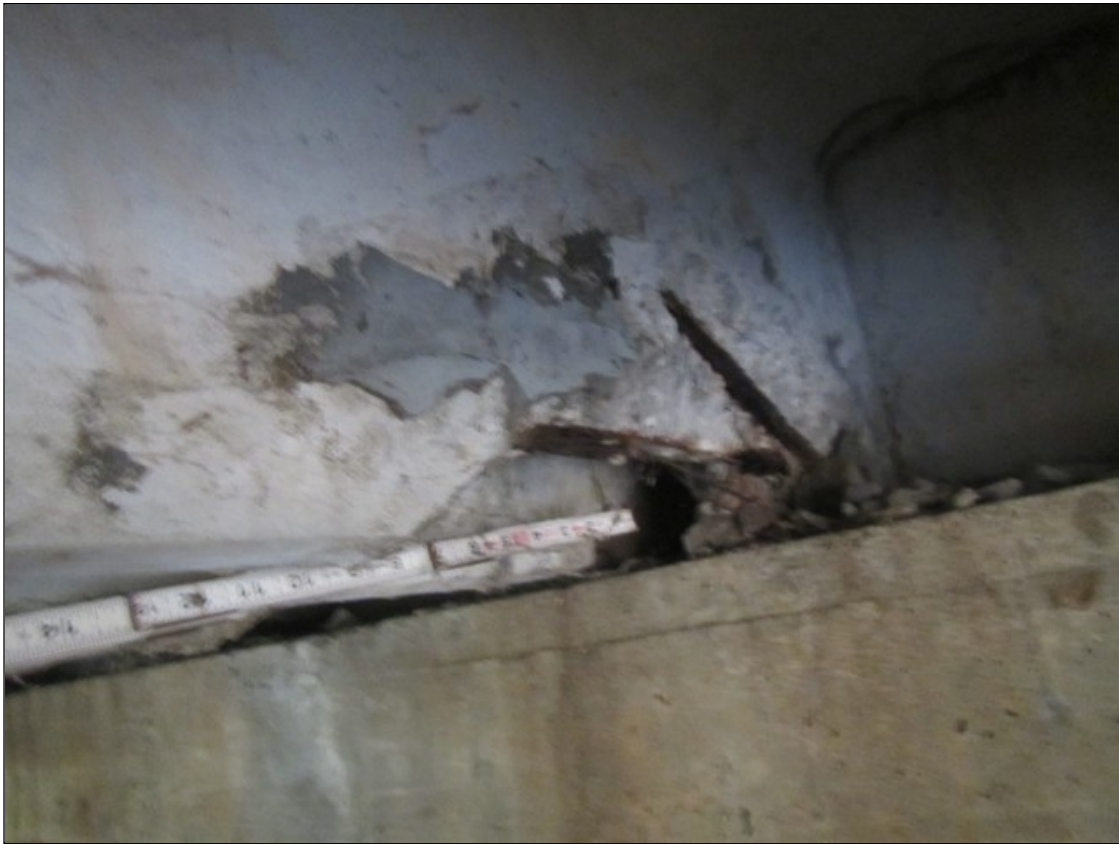
Span 1 Slab 10: MUNICIPAL PAR: 20 INCH X 3 INCH X 9 INCH SPALL WITH EXPOSED REBAR AND BROKEN STRAND IN LEG 2 AT ABUTMENT 1
