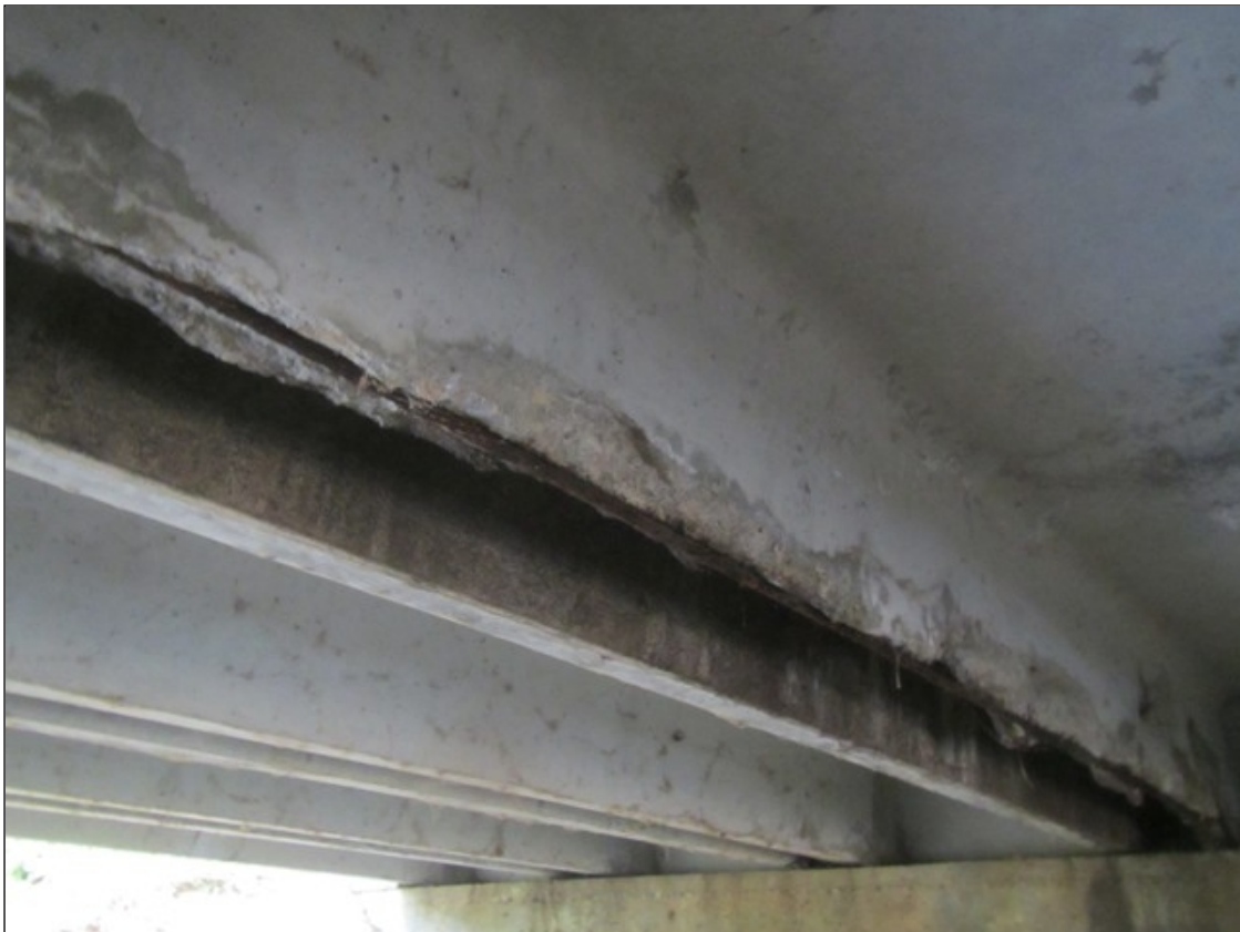
Span 1 Slab 16: MUNICIPAL PAR: 108 INCH X 3 INCH X 5 INCH SPALL WITH EXPOSED REBAR AND STRAND WITH 80% REMAINING IN LEG 2 EXTENDING FROM ABUTMENT 1
