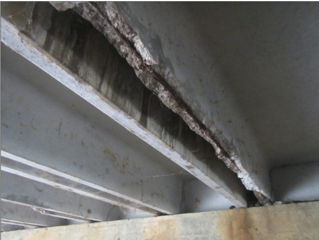
Span 1 Slab 6: MUNICIPAL PAR: 82 INCH X 3 INCH X 4 INCH SPALL WITH EXPOSED REBAR AND STRAND IN LEG 1 EXTENDING FROM ABUTMENT 2
