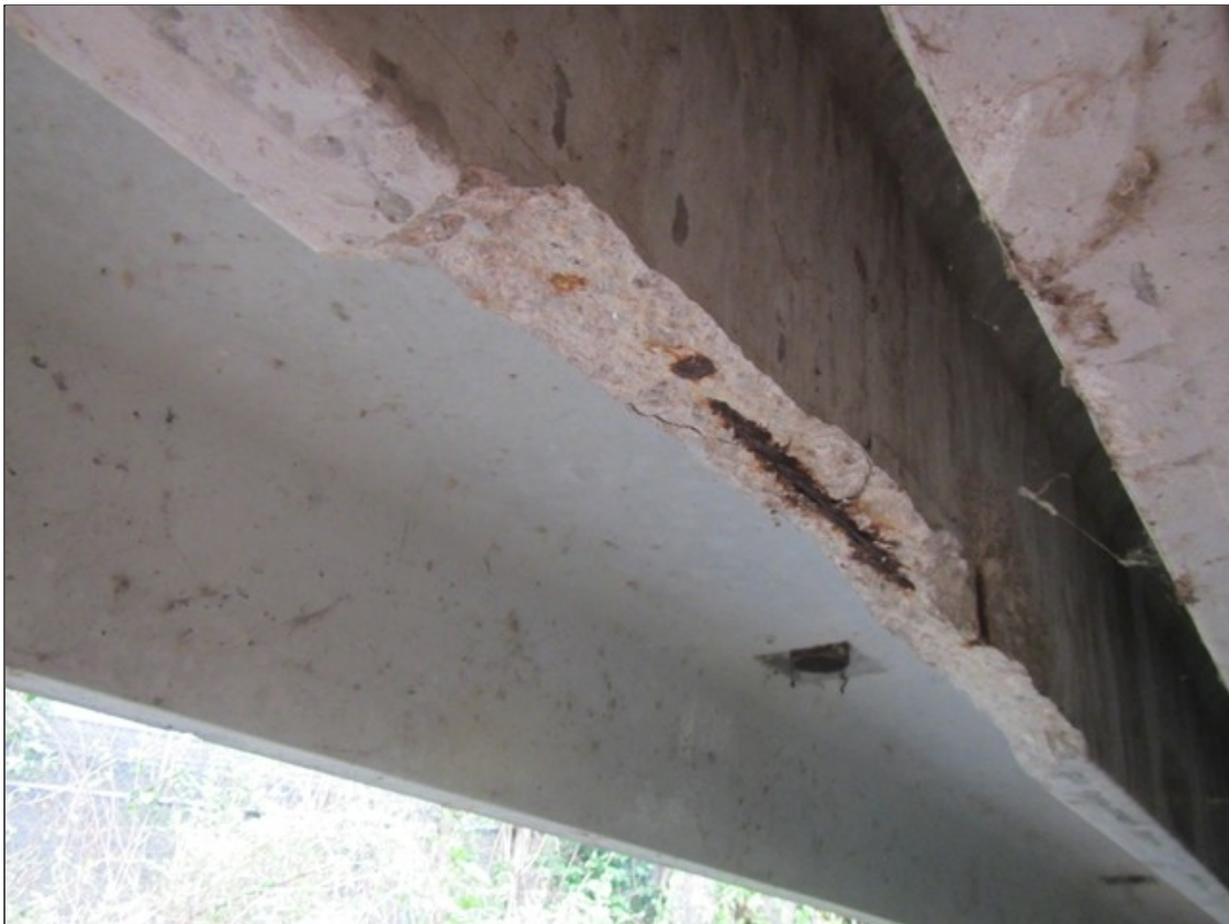
Span 1 Slab 19: MUNICIPAL PAR: 36 INCH X 3 INCH X 3 INCH SPALL WITH EXPOSED REBAR AND STRAND IN LEG 1, APPROXIMATELY 8 FEET FROM ABUTMENT 2
