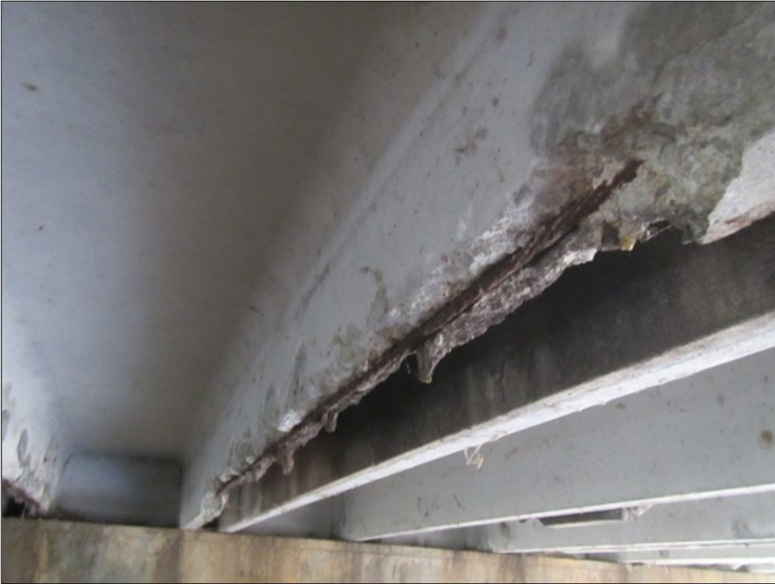
Span 1 Slab 6: MUNICIPAL PAR: 81 INCH X 3 INCH X 3 INCH SPALL WITH EXPOSED REBAR AND STRAND IN LEG 1, APPROXIMATELY 5 FOOT FROM ABUTMENT 1
