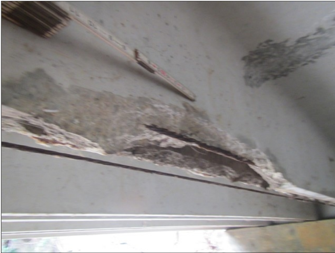
Span 1 Slab 4: MUNICIPAL PAR: 36 INCH X 3 INCH X 5 INCH SPALL WITH EXPOSED REBAR AND STRAND IN LEG 1 NEAR MIDSPAN
