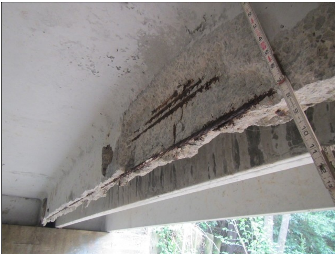
Span 1 Slab 2: MUNICIPAL PAR: 150 INCH X 3 INCH X 10 INCH SPALL WITH EXPOSED REBAR AND STRANDS WITH 20 INCH X 8 INCH SPALL WITH 4 EXPOSED STRANDS IN LEG 1 EXTENDING FROM ABUTMENT 1 AT MIDSPAN
