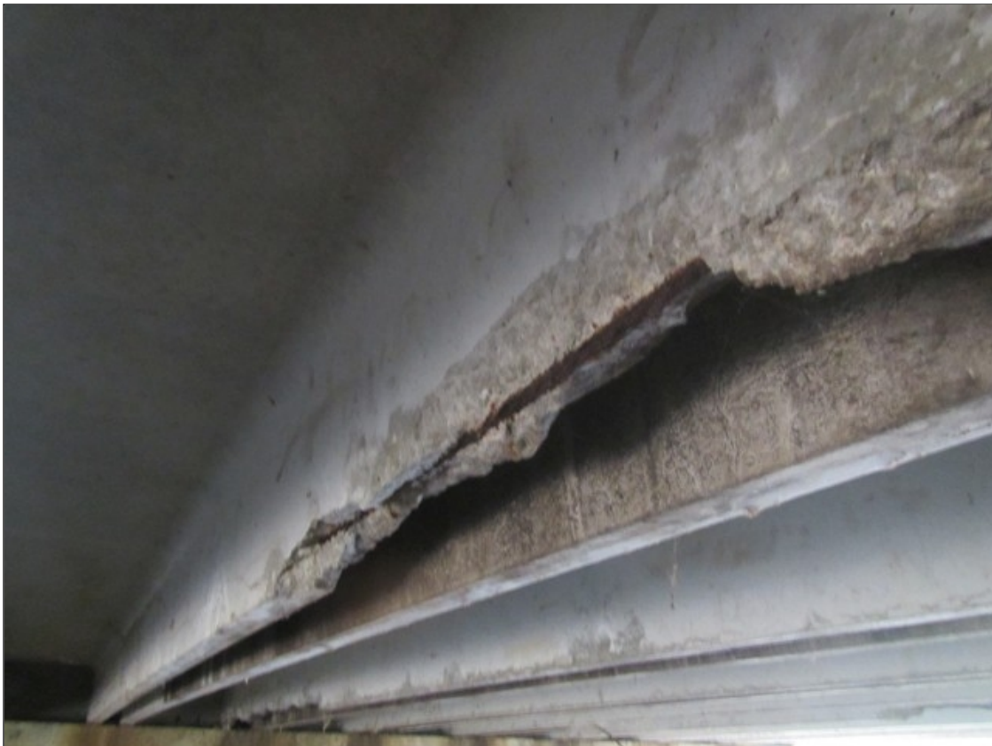
Span 1 Slab 12: MUNICIPAL PAR: 55 INCH X 3 INCH X 4 INCH SPALL WITH EXPOSED REBAR AND 80% REMAINING IN STRAND IN LEG 2 NEAR MIDSPAN
