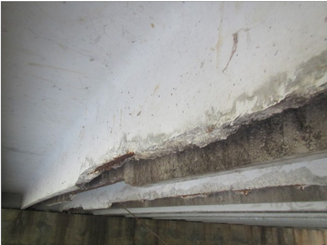
Span 1 Slab 17: MUNICIPAL PAR: 57 INCH X 3 INCH X 4 INCH SPALL WITH EXPOSED REBAR AND STRAND WITH 50% SECTION REMAINING IN LEG 1, APPROXIMATELY 8 FEET FROM ABUTMENT 2
