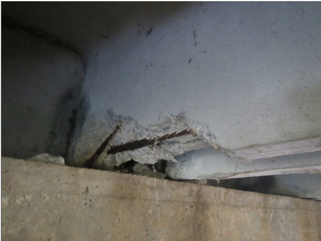
Span 1 Slab 10: MUNICIPAL PAR: 19 INCH X 3 INCH X 4 INCH SPALL WITH EXPOSED REBAR AND STRAND IN LEG 1 AT ABUTMENT 1
