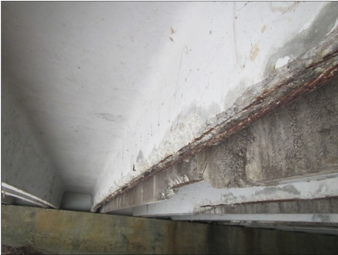
Span 1 Slab 3: MUNICIPAL PAR: 20 FOOT X 3 INCH X 5 INCH SPALL WITH EXPOSED REBAR AND STRAND IN LEG 2, BEGINNING APPROXIMATELY 2 FEET FROM ABUTMENT 2 WITH 80% REMAINING IN EXPOSED STRAND
