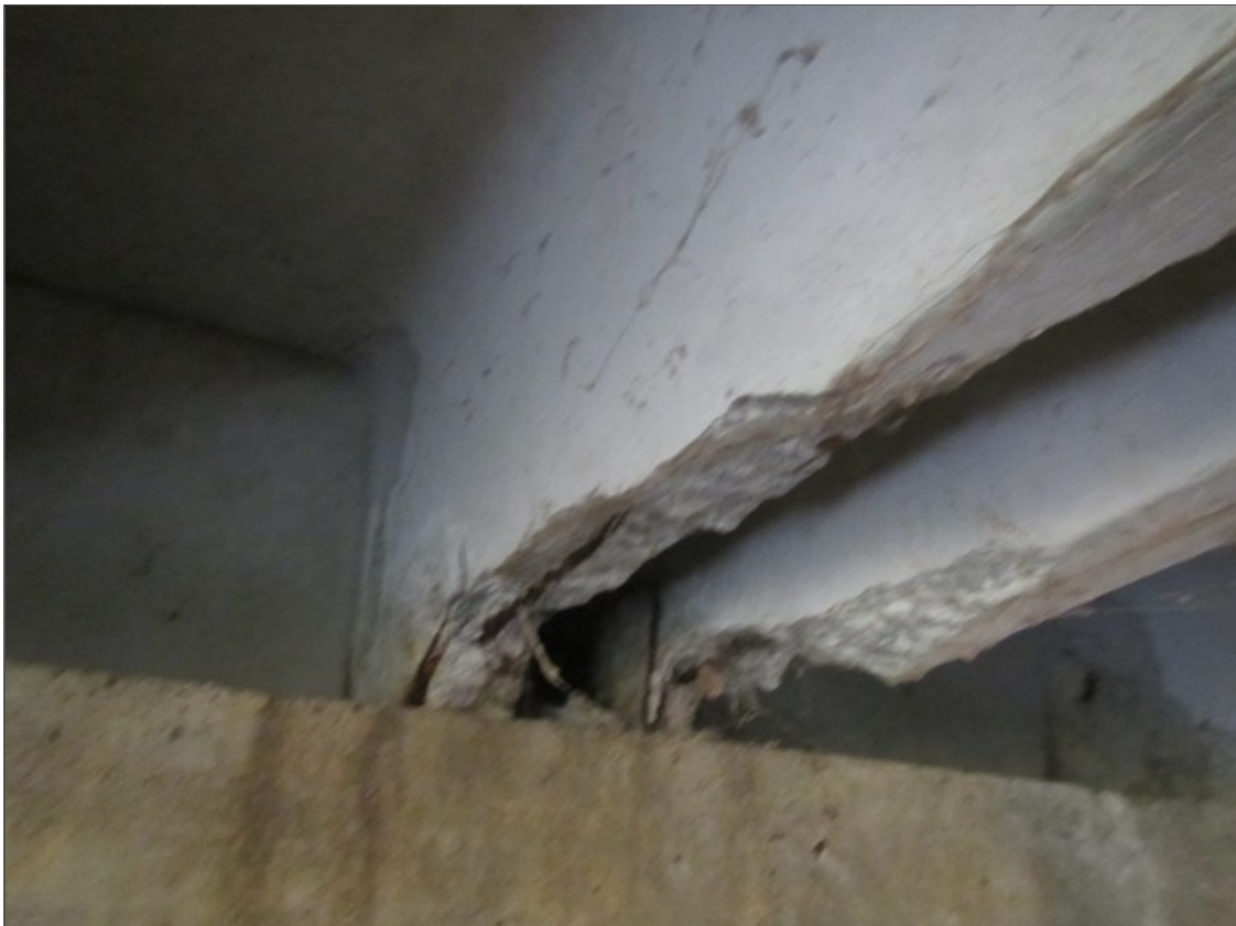
Span 1 Slab 12: MUNICIPAL PAR: 29 INCH X 3 INCH X 4 INCH SPALL WITH EXPOSED REBAR AND STRAND IN LEG 1 AT ABUTMENT 1
