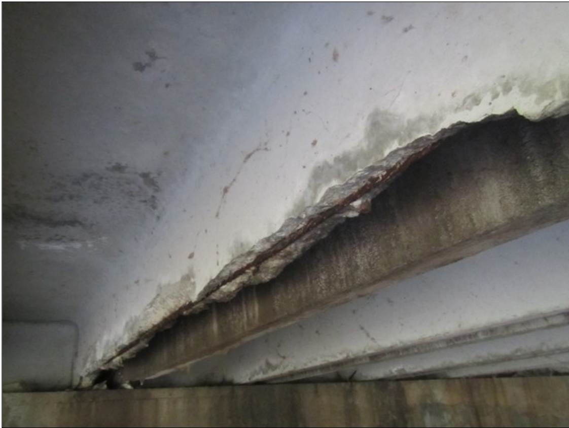
Span 1 Slab 16: MUNICIPAL PAR: 96 INCH X 3 INCH X 4 INCH SPALL WITH EXPOSED REBAR AND STRAND IN LEG 1 EXTENDING FROM ABUTMENT 1
