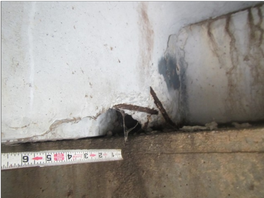
Span 1 Slab 3: MUNICIPAL PAR: 22 INCH X 3 INCH X 6 INCH SPALL WITH EXPOSED REBAR AND STRAND IN LEG 2 AT ABUTMENT 1
