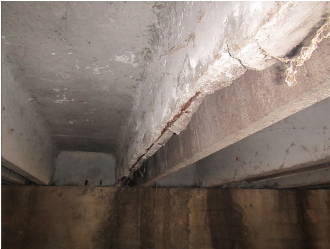
Span 1 Slab 13: MUNICIPAL PAR: 84 INCH X 3 INCH X 4 INCH SPALL WITH EXPOSED REBAR AND STRAND IN LEG 2 EXTENDING FROM ABUTMENT 2
