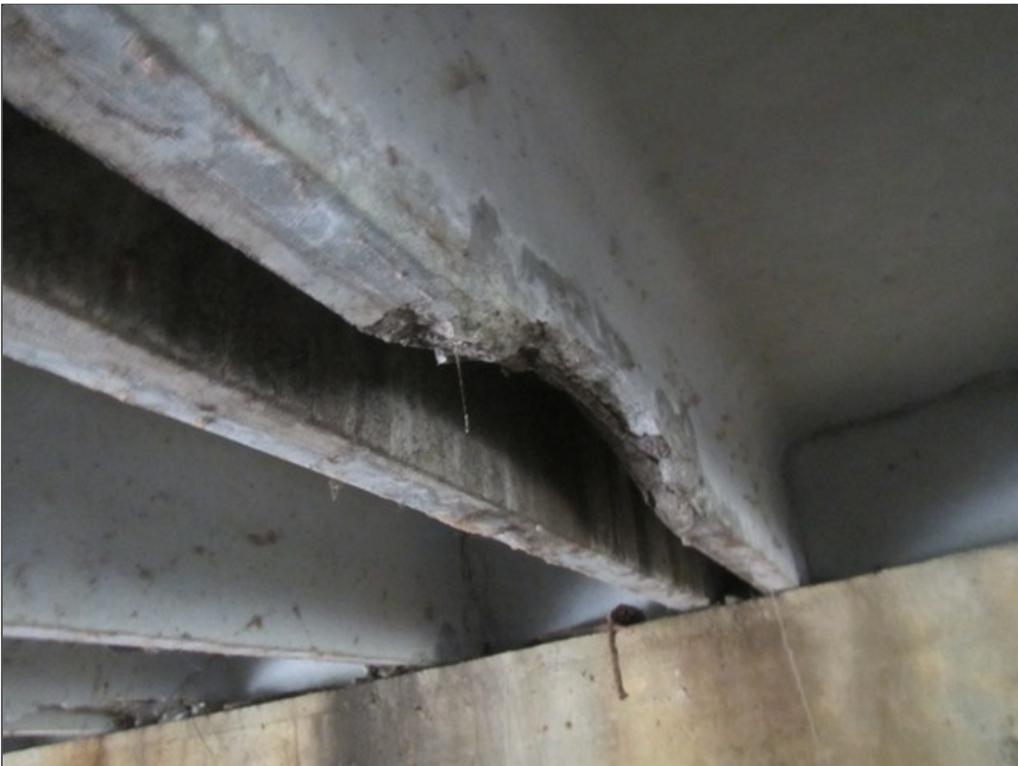
Span 1 Slab 8: MUNICIPAL PAR: 27 INCH X 3 INCH X 4 INCH SPALL WITH EXPOSED REBAR AND STRAND IN LEG 1, APPROXIMATELY 3 FEET FROM ABUTMENT 2
