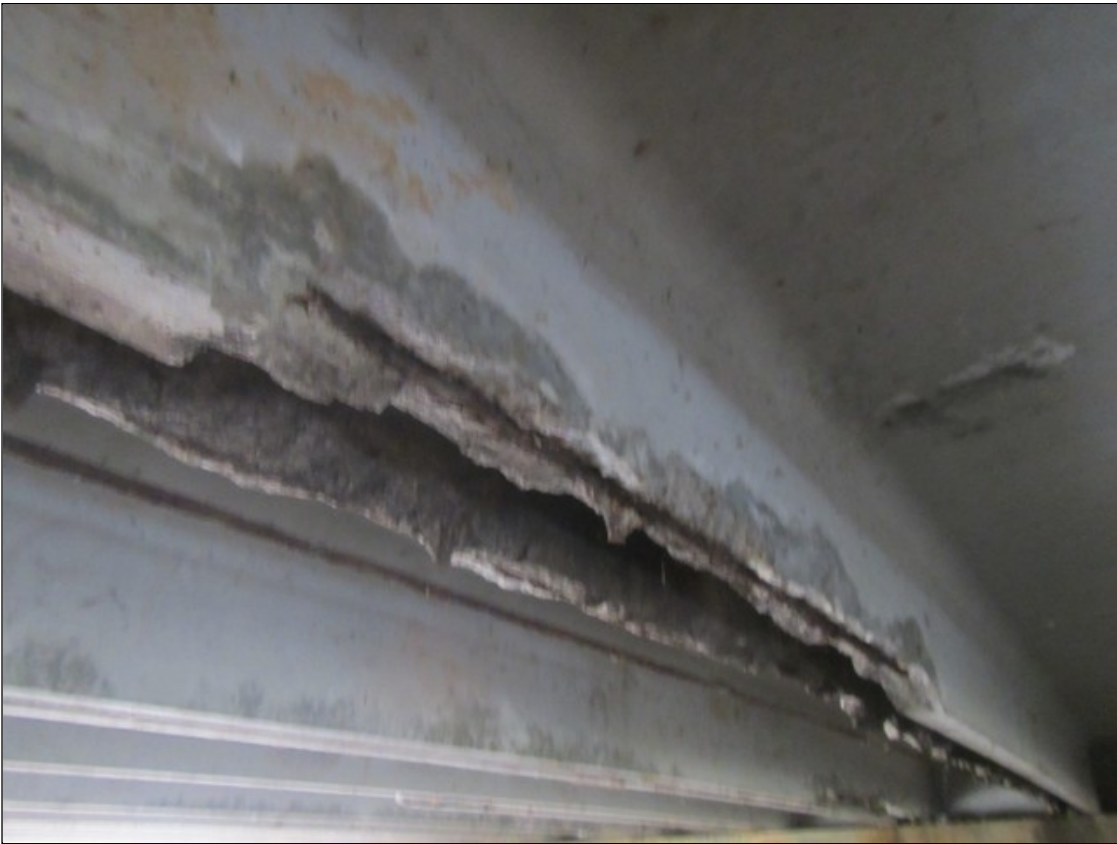
Span 1 Slab 7: MUNICIPAL PAR: 58 INCH X 3 INCH X 3 INCH SPALL WITH EXPOSED REBAR AND STRAND IN LEG 1 AT MIDSPAN
