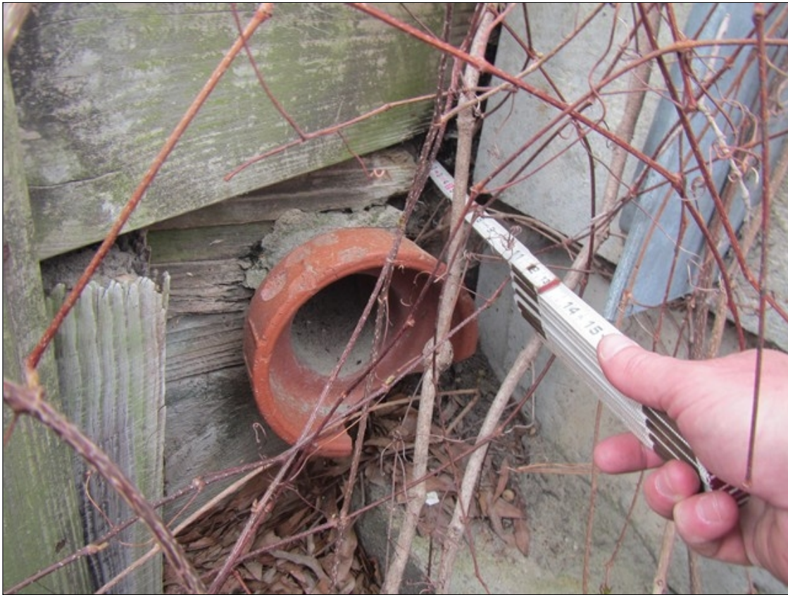
MUNICIPAL PAR: 15 INCH X 6 INCH X FULL DEPTH AREA OF DECAY WITH EXPOSED FILL IN FACE OF SOUTHWEST WINGWALL ADJACENT TO UNIT 1
