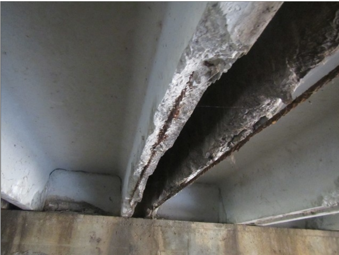
Span 1 Slab 7: MUNICIPAL PAR: 63 INCH X 3 INCH X 3 INCH SPALL WITH EXPOSED REBAR AND STRAND IN LEG 1 EXTENDING FROM ABUTMENT 1
