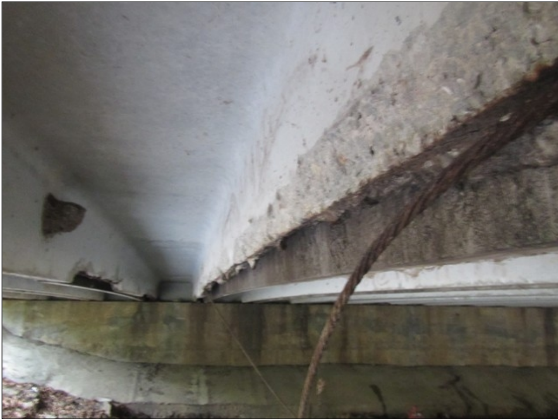
Span 1 Slab 16: MUNICIPAL PAR: 14 FOOT X 3 INCH X 6 INCH SPALL WITH EXPOSED REBAR WITH SEVERED STRAND IN LEG 1 BEGINNING APPROXIMATELY 4 FOOT FROM ABUTMENT 2 TO MIDSPAN
