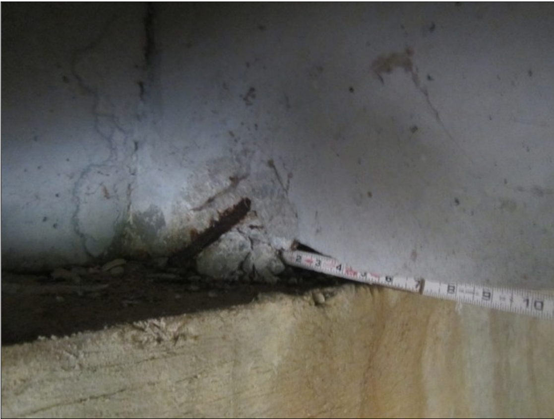
Span 1 Slab 8: MUNICIPAL PAR: 8 INCH X 4 INCH X UP TO FULL DEPTH SPALLS WITH EXPOSED REBAR ON BOTH LEGS AT ABUTMENT 2
