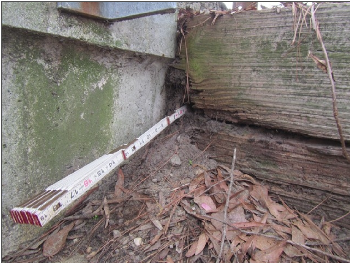
MUNICIPAL PAR: 11 INCH X 10 INCH X FULL DEPTH AREA OF DECAY WITH EXPOSED FILL IN FACE OF NORTHWEST WINGWALL ADJACENT TO UNIT 19
