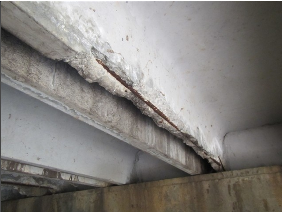
Span 1 Slab 4: MUNICIPAL PAR: 63 INCH X 3 INCH X 4 INCH SPALL WITH EXPOSED REBAR AND STRAND IN LEG 2 EXTENDING FROM ABUTMENT 1
