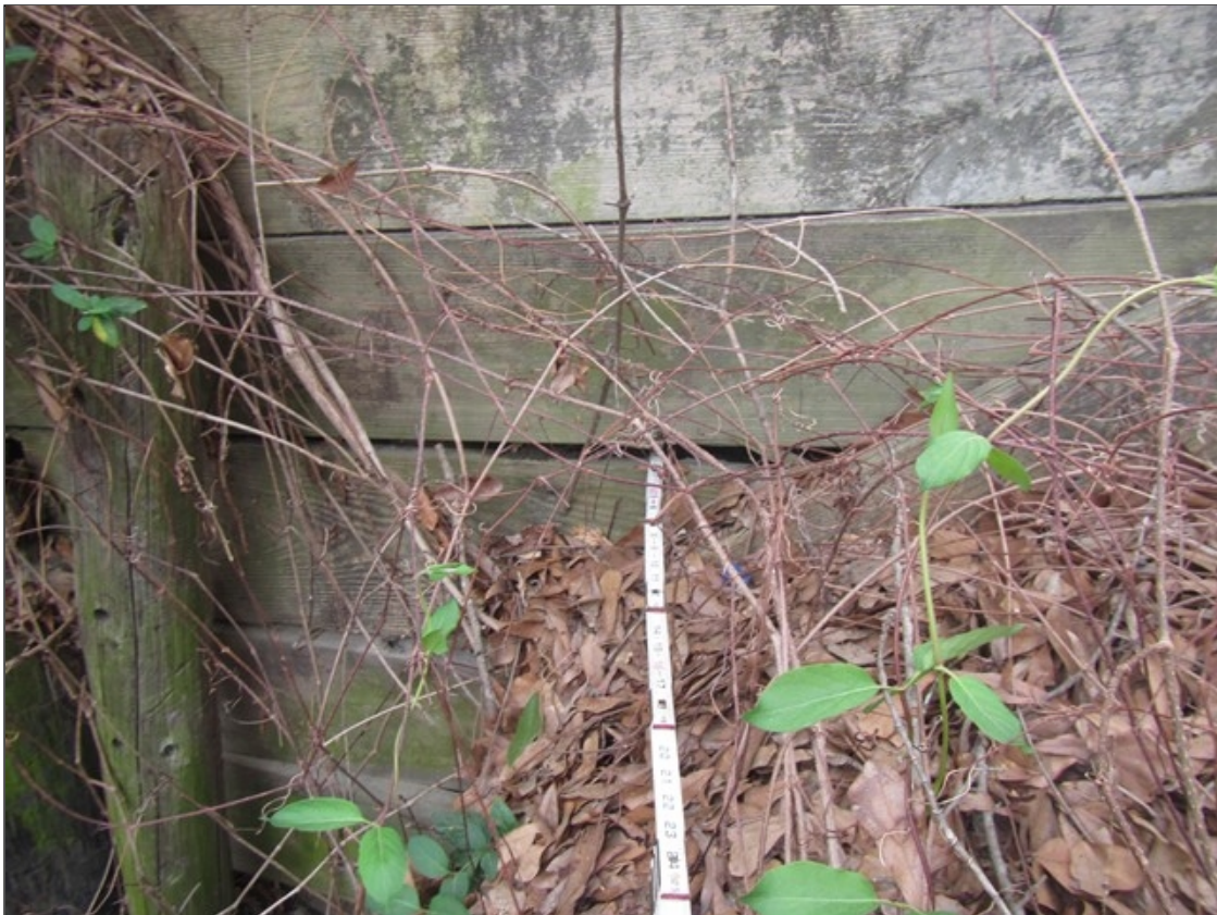
MUNICIPAL PAR: 4 FEET SECTION WITH UP TO 1 INCH GAPS WITH EXPOSED FILL IN FACE OF SOUTHWEST WINGWALL TO LEFT OF STORM DRAIN INLET
