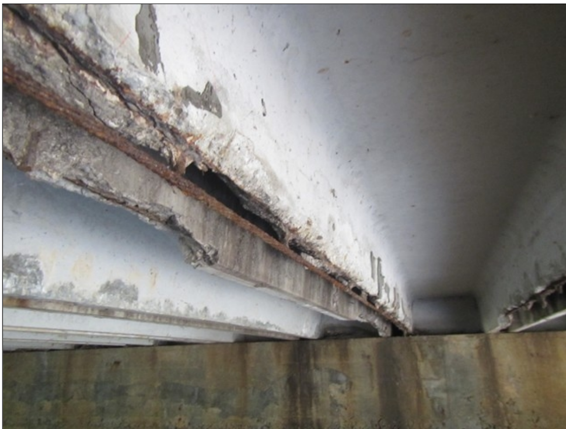
Span 1 Slab 6: MUNICIPAL PAR: 30 FOOT X 3 INCH X 9 INCH SPALL WITH EXPOSED STRAND WITH UP TO 50% LOSS IN STRAND WITH AN ADDITIONAL 30 INCH X 6 INCH X 2 INCH DEEP SPALL AT MIDSPAN WITH A SECOND EXPOSED STRAND WITH 90% SECTION REMAINING
