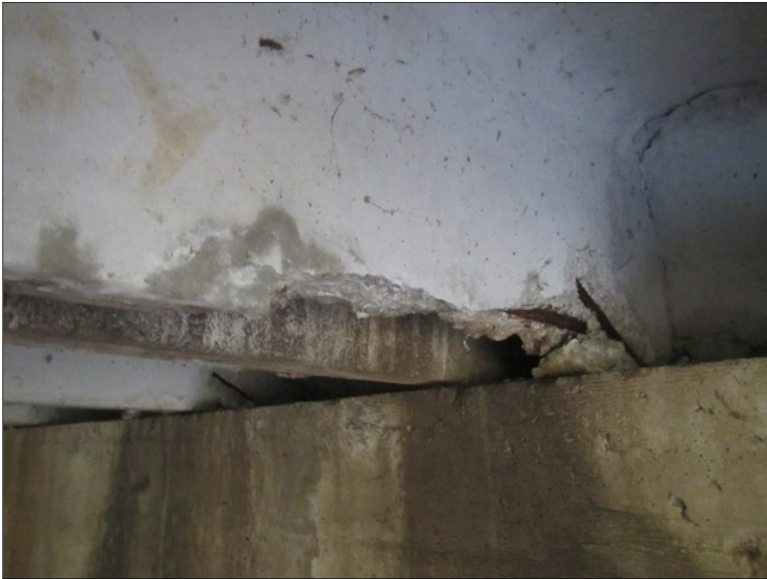
Span 1 Slab 15: MUNICIPAL PAR: 24 INCH X 3 INCH X 5 INCH SPALL WITH EXPOSED REBAR AND STRAND IN LEG 1 EXTENDING FROM ABUTMENT 2
