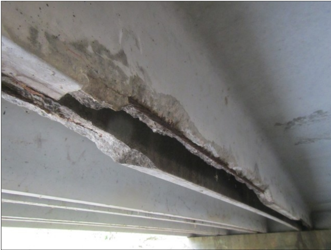
Span 1 Slab 16: MUNICIPAL PAR: 60 INCH X 3 INCH X 4 INCH SPALL WITH EXPOSED REBAR AND STRAND WITH 80% REMAINING IN LEG 2 NEAR MIDSPAN
