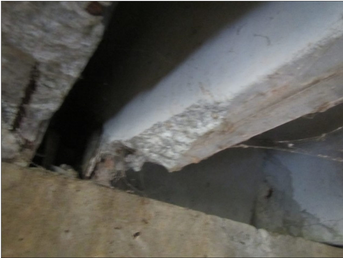
Span 1 Slab 11: MUNICIPAL PAR: 20 INCH X 3 INCH X 4 INCH SPALL WITH EXPOSED REBAR AND STRAND IN LEG 2 AT ABUTMENT 1
