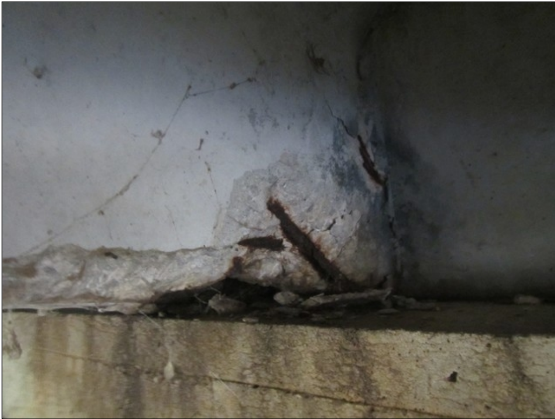
Span 1 Slab 12: MUNICIPAL PAR: 24 INCH X 3 INCH X 5 INCH SPALL WITH EXPOSED REBAR AND STRAND IN LEG 2 AT ABUTMENT 1
