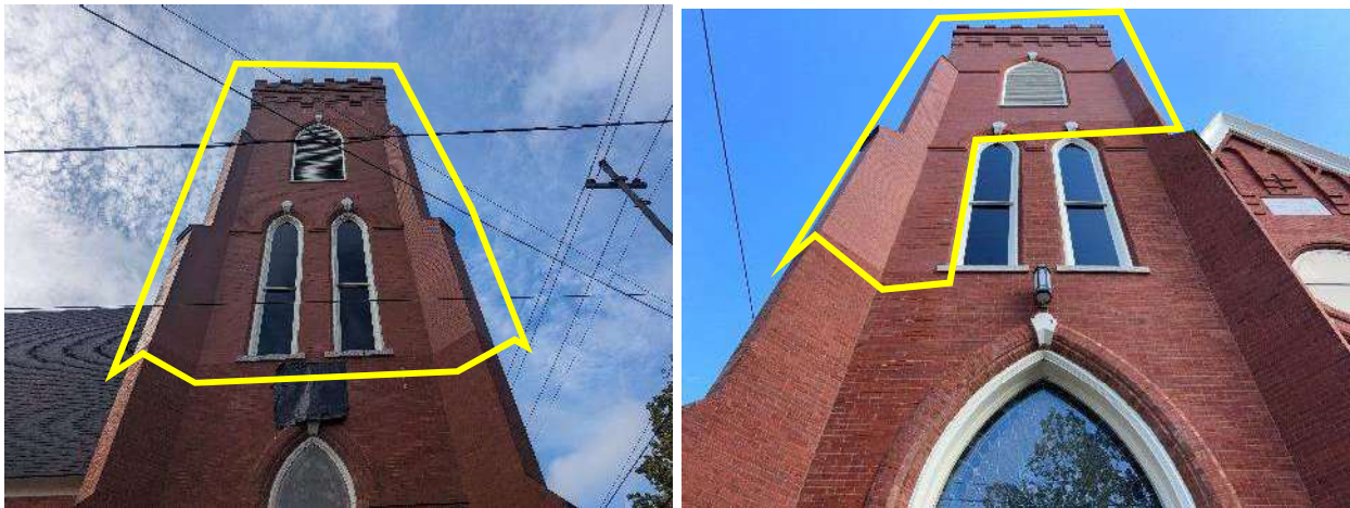
New Brick (Highlighted) Installed Above Old Brick at North (Left) and West (Right) Elevation
