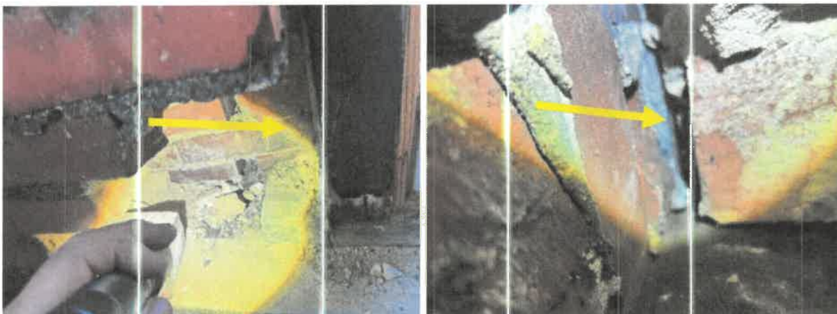
Large Gap or Separation Present Between Interior Brick Wythe and Exterior Brick Wythe
