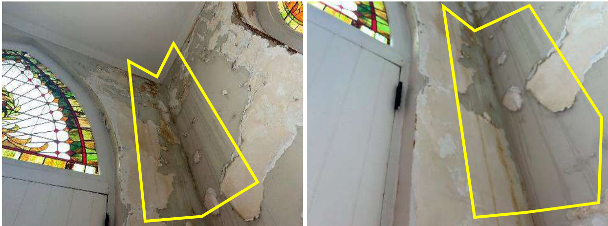
Water Streaming Down Wall Below Area Where Exterior Spray Rack Installed
