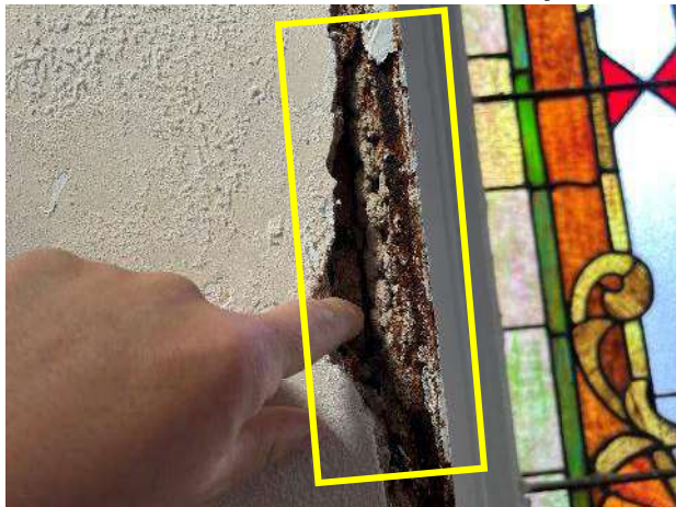
Damaged Plaster at the Corner
