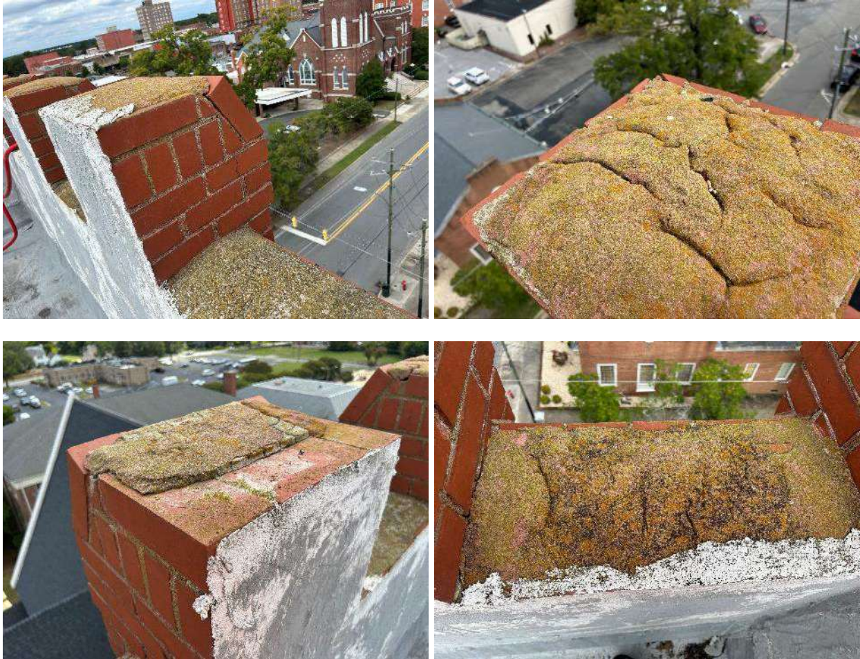
Deteriorated Mortar on Battlement
