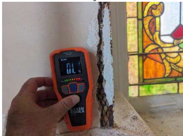
Elevated Moisture Reading
