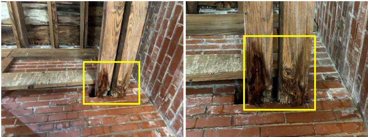
Wet, Deteriorated Wood Beams Set in Brick Masonry Beam Pockets
