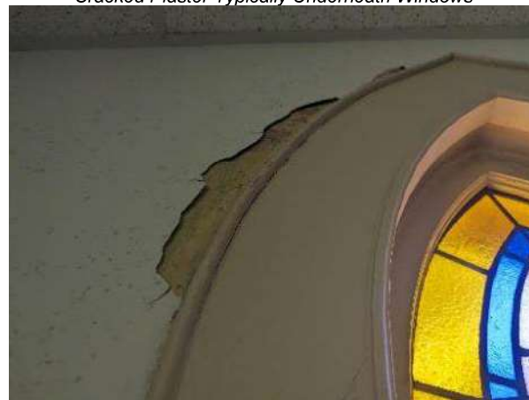
Damaged Finishes Adjacent Window Head
