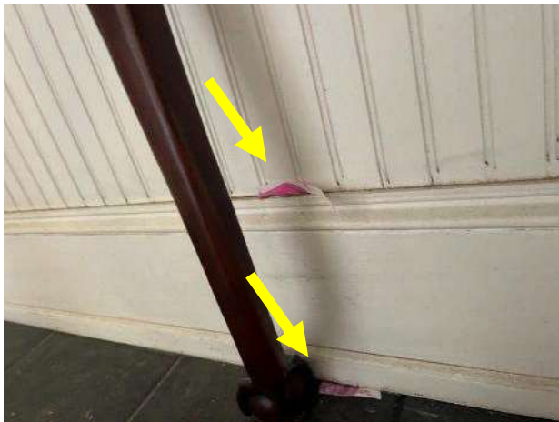
Water Infiltration along Interior of Paneling
