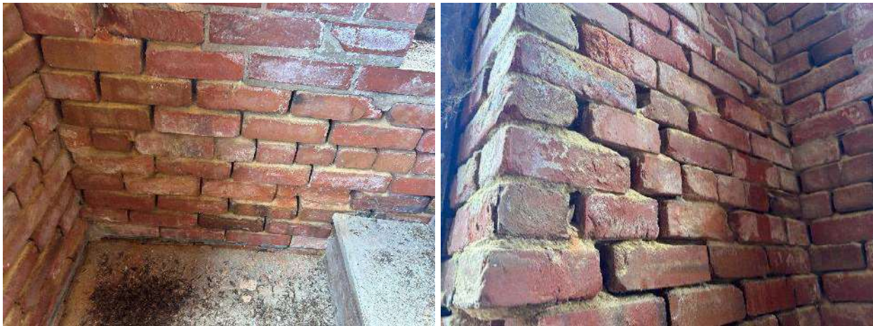
Significant Mortar Deterioration
