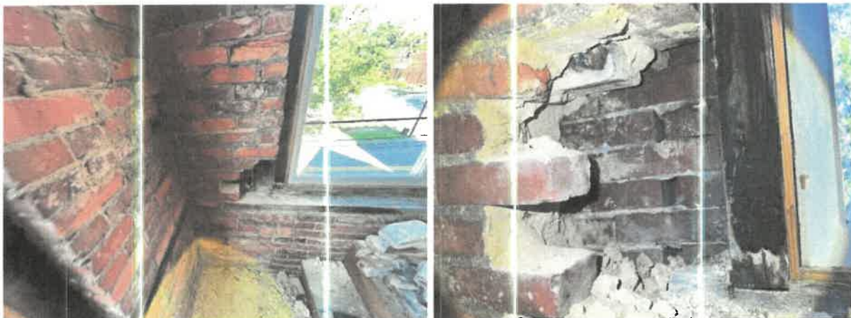
No Skewed Header or Visible Attachment Between Brick Units
