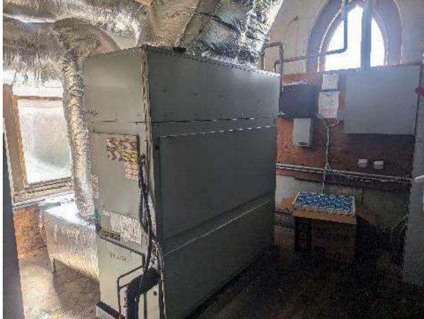
Second Floor Mechanical Room
