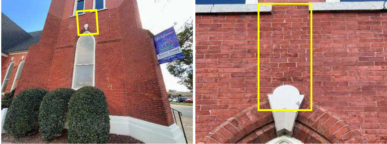
Crack Along North Elevation of Tower
