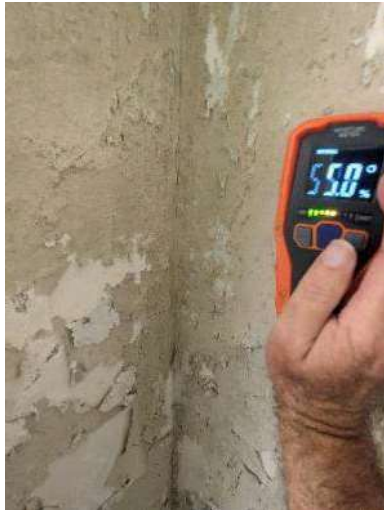
Elevated Moisture Reading Along Interior Side of Plaster.
