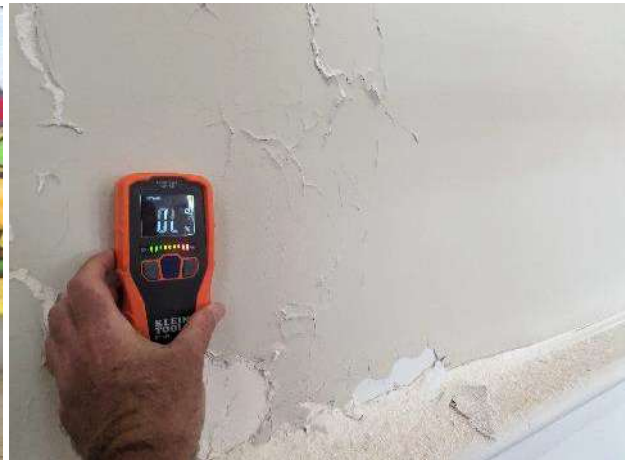
Elevated Moisture Reading
