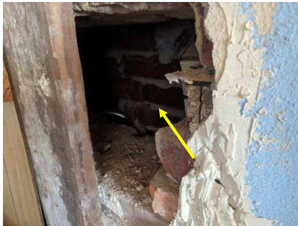
Gap in brick masonry
