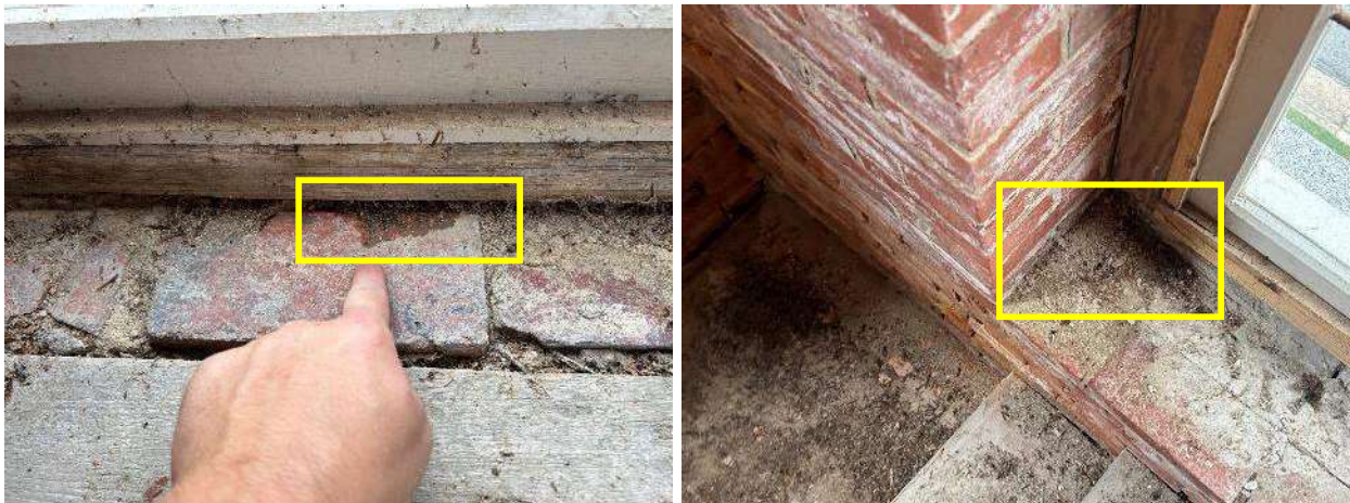
Water Pooling on West Sill (Left) and North Sill (Right)
