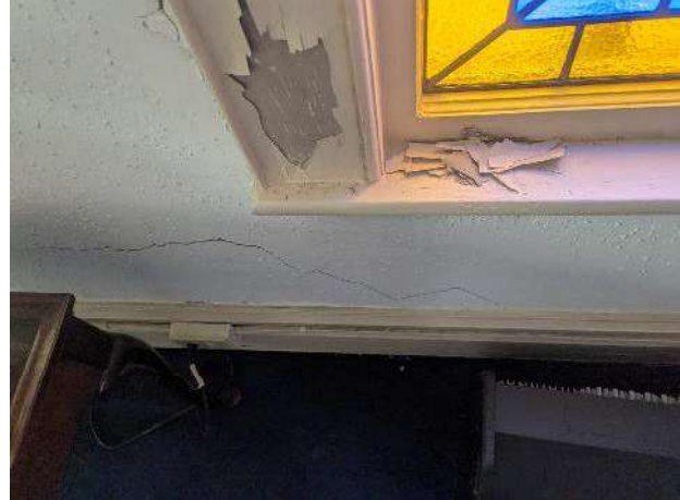
Trim Paint Delamination
