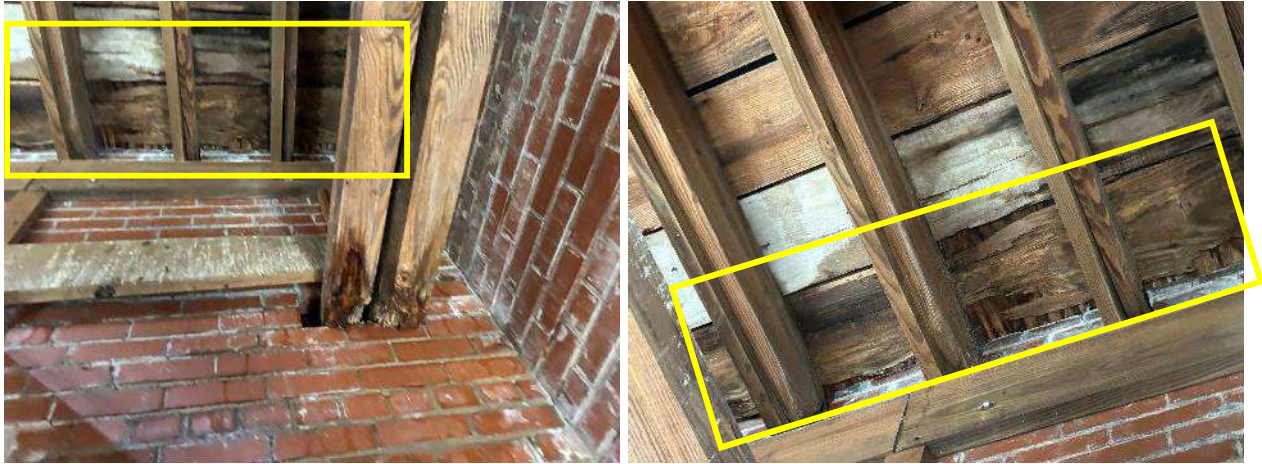
Significantly Deteriorated Wood Roof Decking Above Leakage Location
