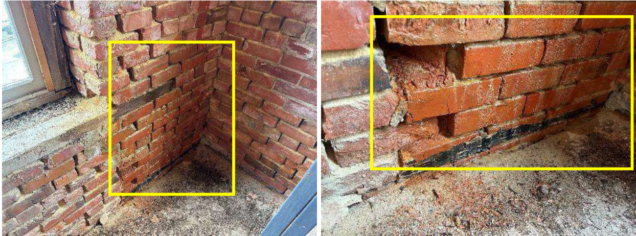
Water Leaking Through Deteriorated Mortar
