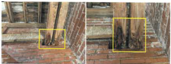
Wet, Deteriorated Wood Beams Set in Brick Masonry Beam Pockets
