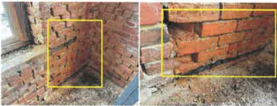
Water Leaking Through Deteriorated Mortar
