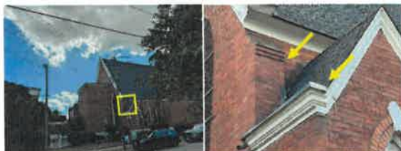
Plaster Extends Beyond Wall Causing Water at Corner, Internal Gutter is Present
