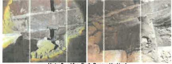
Mortar Crumbling, Easily Removed by Hand
