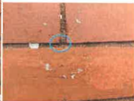
Rilem Test Tube - Test #5 - 4.5ml Absorbed in Less than 1-Minute with Small Void in Mortar Visible.
