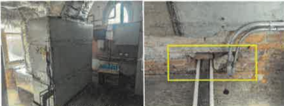
Second Floor Mechanical Room
