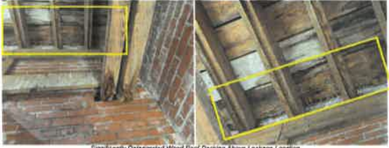
Significantly Deteriorated Wood Floor Decking Above Leakage Location
