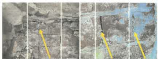
Daylight Visible Through Exterior Mortar
