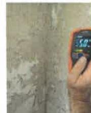
Elevated Moisture Reading Along Interior Side of Plaster.
