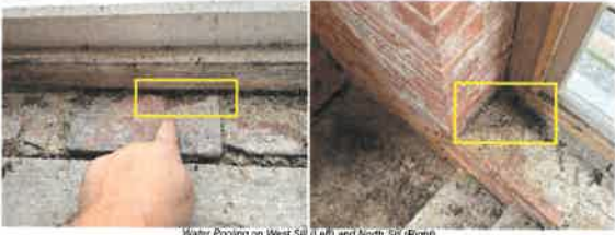
Water Pooling on West Sill (Left) and North Sill (Right)
