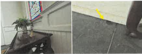
Water Infiltration Noted at Two (2) Locations Below Window Area
