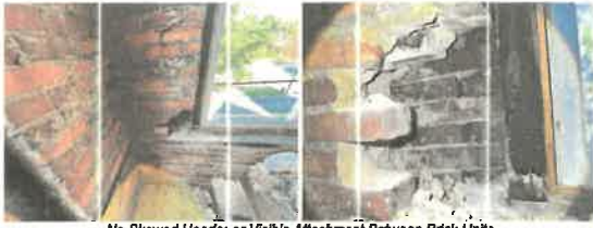
No Skewed Header or Visible Attachment Between Brick Units
