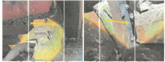
Large Gap or Separation Present Between Interior Brick Wythe and Exterior Brick Wythe
