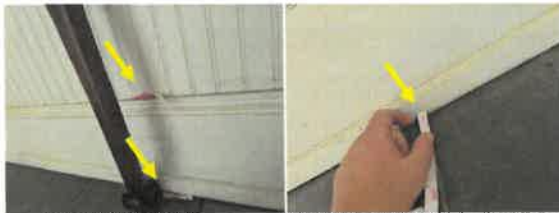
Water Infiltration along Interior of Paneling
