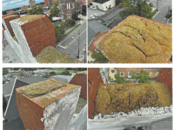
Deteriorated Mortar on Battlement
