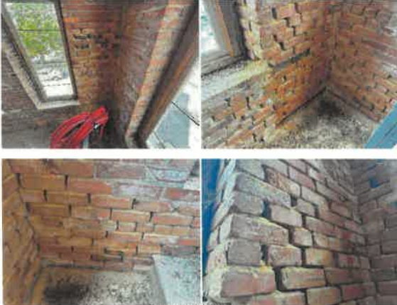
Significant Mortar Deterioration
