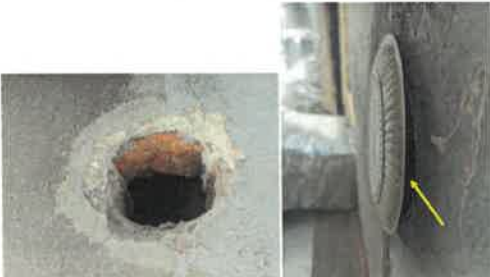
Abandoned Penetrations of Brick Masonry Wall
