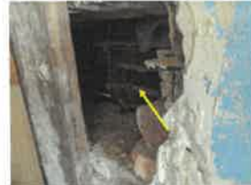
Gap in brick masonry
